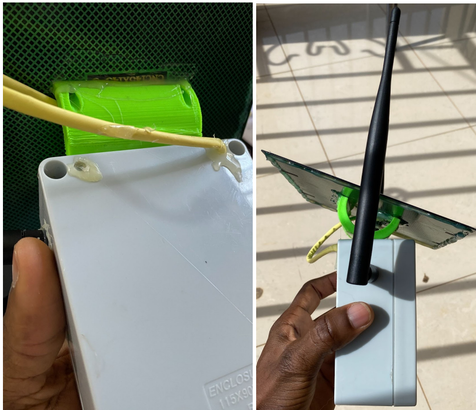
Figure 24 – solar panel inclined at 25-38 degrees with cable protected by heat shrink tube
